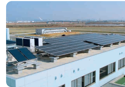
Generating capacity : 28.2 kW
