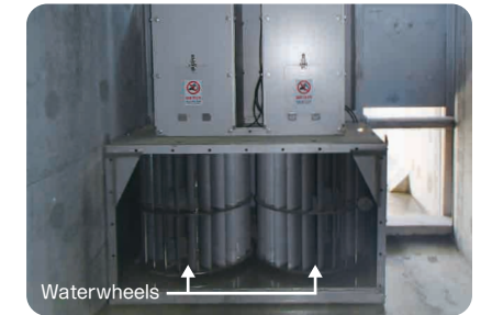
Generating capacity : 7.5 kW
