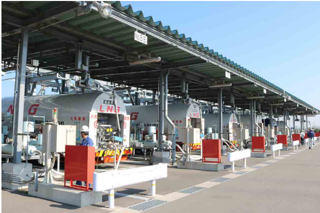
LNG tank truck loading facilities
